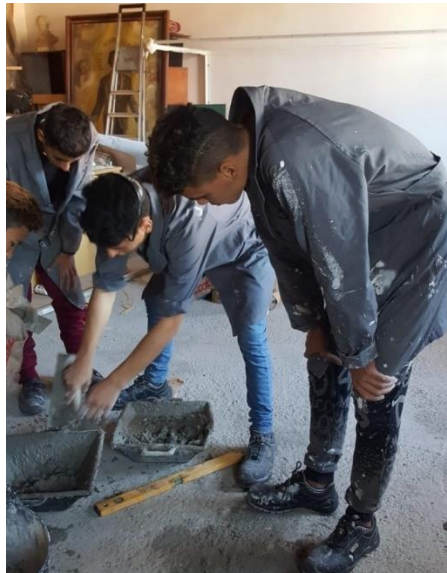
Young people being trained to renovate a vacant flat in Mataro, Spain © Yes We Rent!
